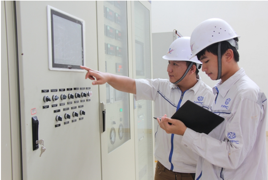
Local workers monitor the operation of generating units at the Nam Phay hydropower station. (Photo: People's Daily/Sun Guangyong)
